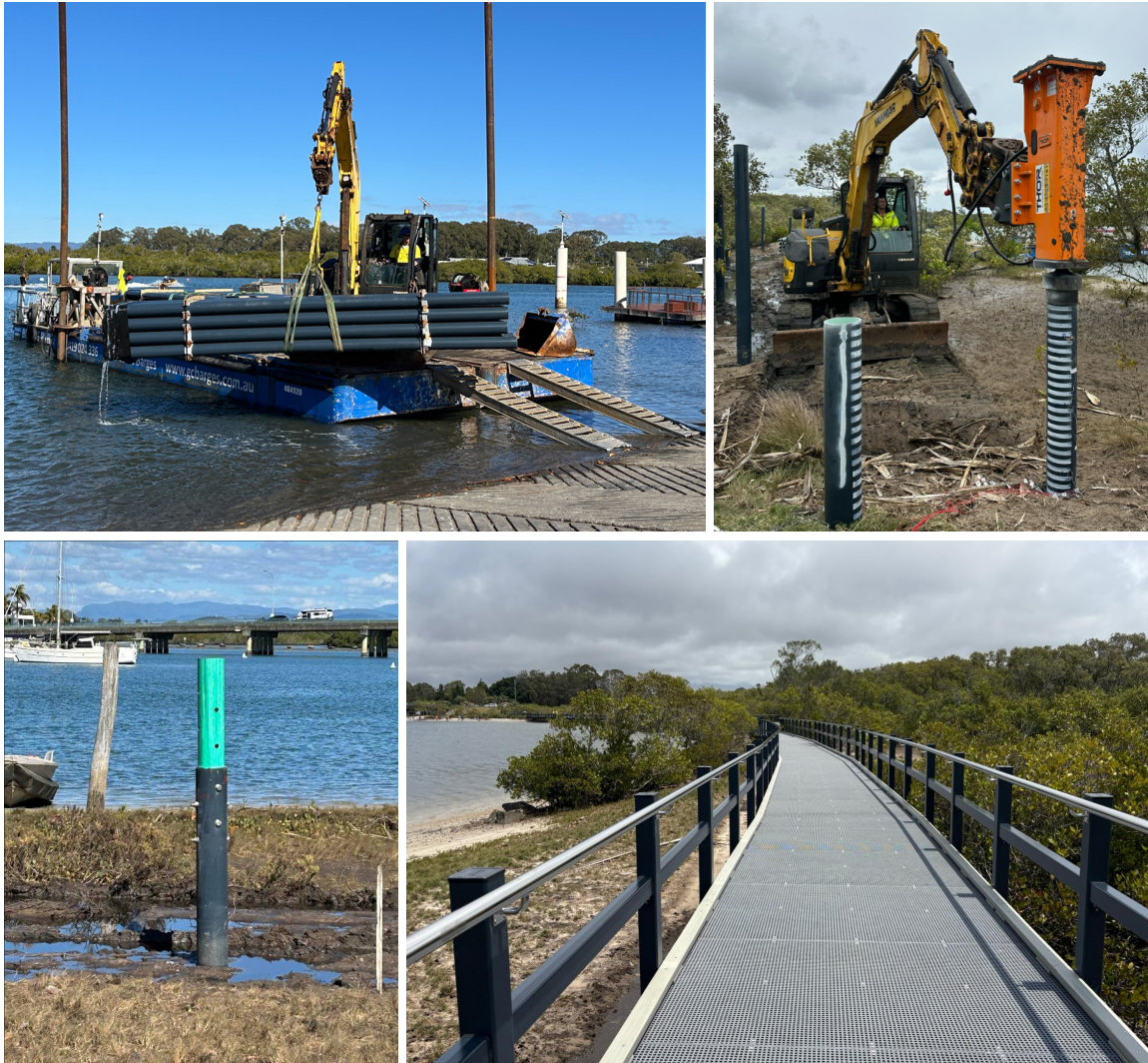
Figure 5. Transport and Install of FRP Piles at Phill Hill Boardwalk and Phill Hill FRP Boardwalk, Gold Coast
