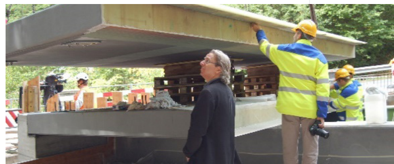
Figure 3. Avançon Bridge, October 2012: Adhesive bonding of composite-balsa sandwich bridge deck onto steel girders, panels with transverse scarf joints in face sheets.
