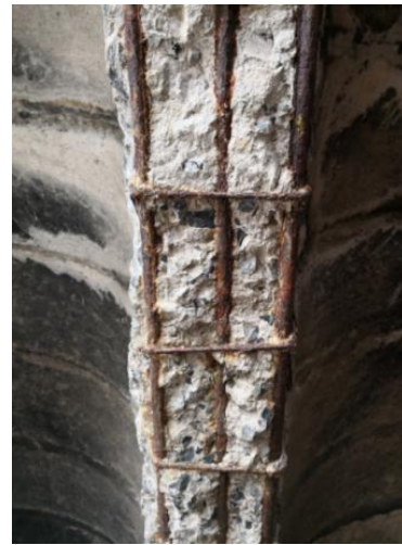
(b) steel bar corrosion
