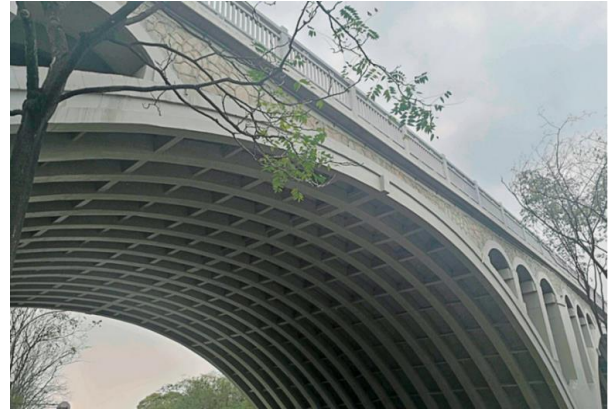
(b) after strengthening
