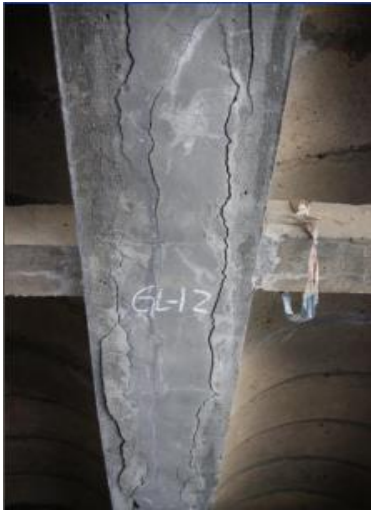
(a) concrete cracking and peeling
