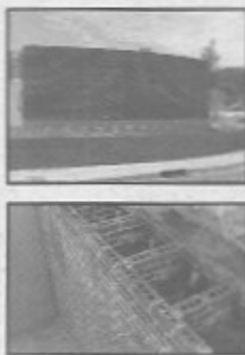
Figure 10: FRP post-tensioned walls at the University of Calgary
