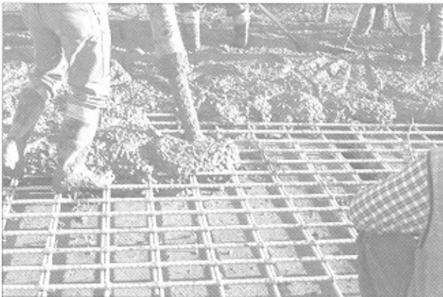
Figure 16: Workers place the bridge deck concrete through and over the GFRP-bar mat.
