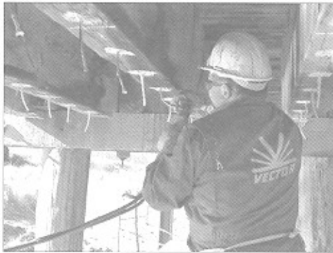
Figure 14: Injection of epoxy resin that provides the bond between the installed GFRP rods and stringers.
