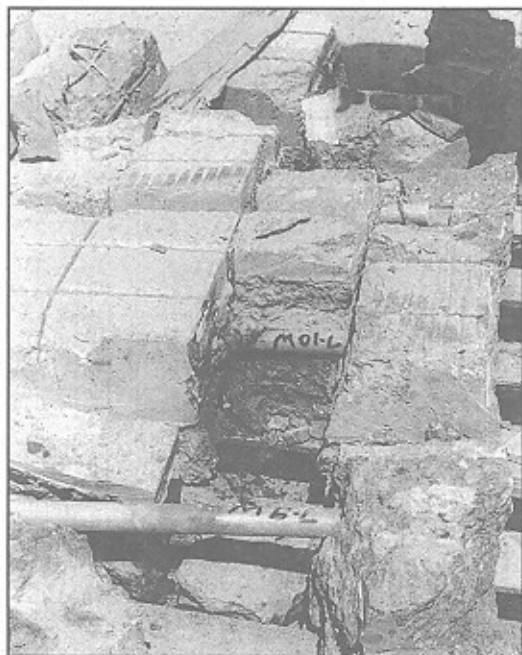
Figure 9. GFRP dowels removed after 13 years of service
