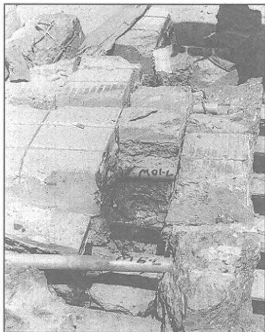
Figure 9. GFRP dowels removed after 13 years of service
