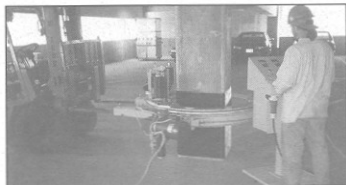
Figure 7. Retrofit of Parking Structures in Salt Lake City, Utah.
