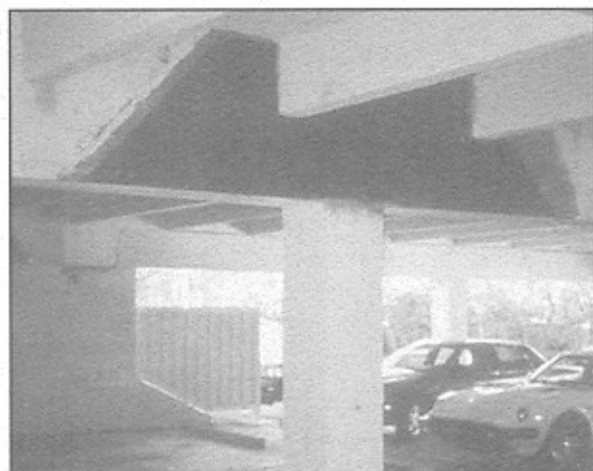
Figure 1. Repair of the main beam for shear strength using Tonen's Forca Tow Sheets.
