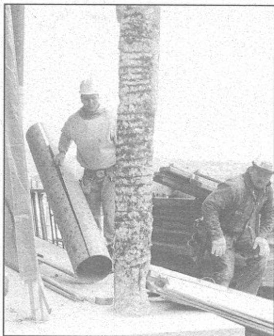
Figure 3a and 3b. Repair of Column at University of Sherbrooke (Before and After)
