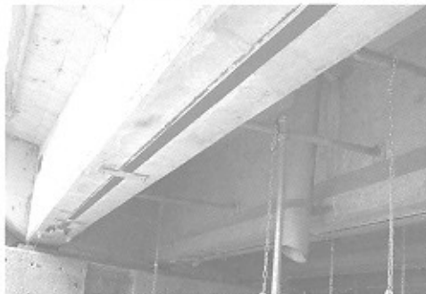
Fig. 1 PC T-girder bridge in Nara Prefecture strengthened by the tensioned CFRP plate method
