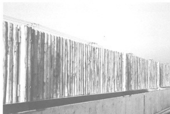
Fig. 5 Wooden sound insulation wall with Technola rods on a highway in Shin-machi, Tokyo
