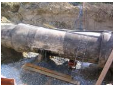
Cracked pipe segment.
