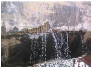
Steel spiral fully corroded at crack.
