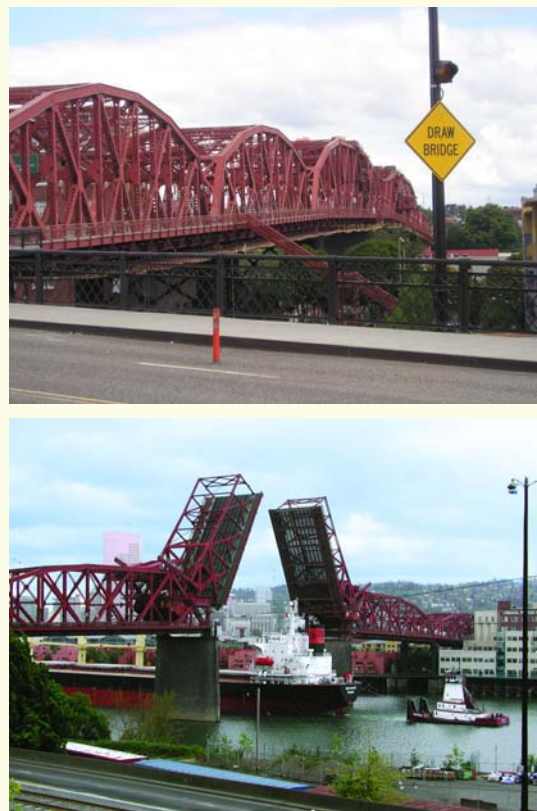
Fig. 1: Vital to Portland’s river and vehicular traffic, the Broadway Bridge’s bascule span utilized a steel grid deck before being replaced by a solid-surface FRP deck in August 2004.
