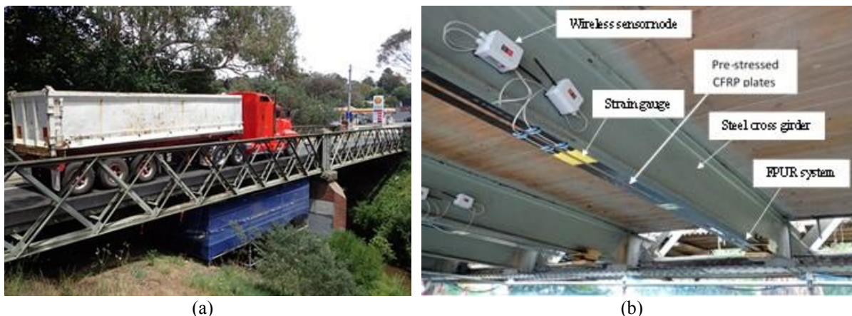
Figure 7. (a) Diamond-Creek Bridge, Melbourne, Australia, (b) application of the FPUR system for CFRP strengthening of the bridge cross-girders (Ghafoori et al. 2018).
